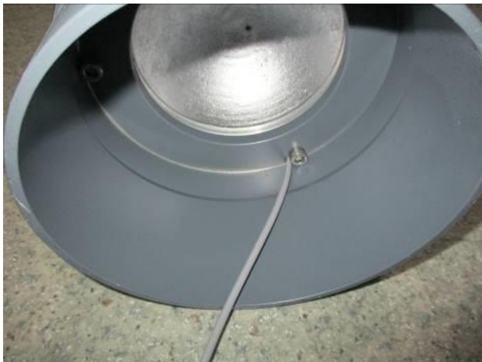
15) Internal wiring where it passes to top side of luminaire and reflector
