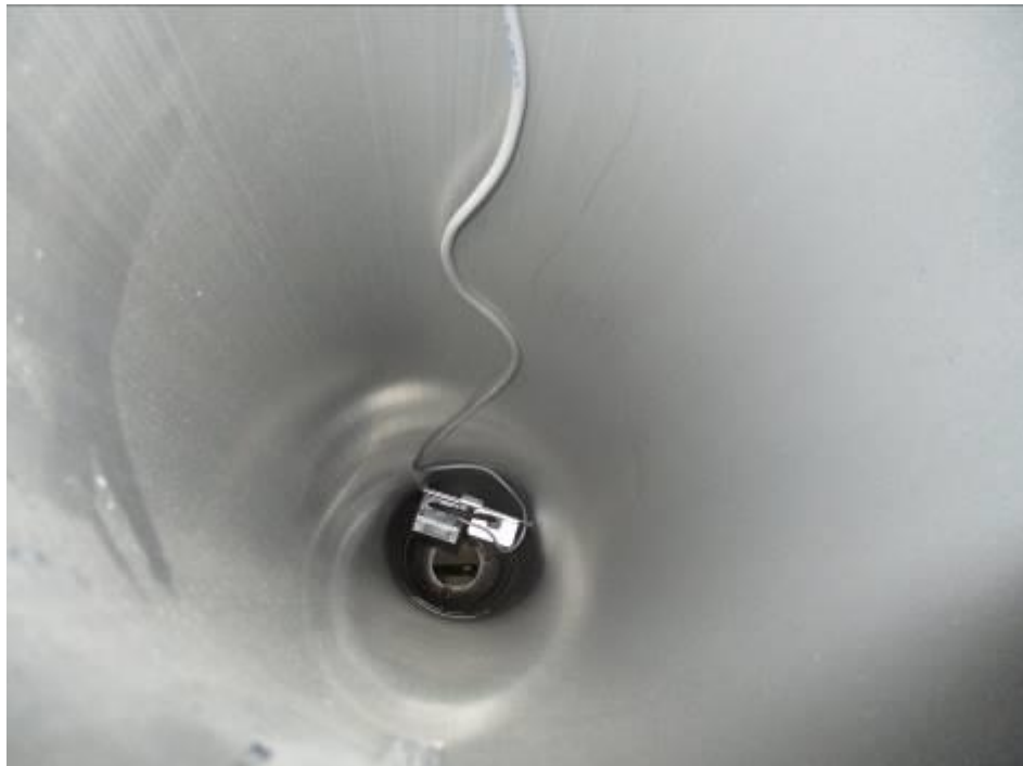
14) Path for internal wiring
